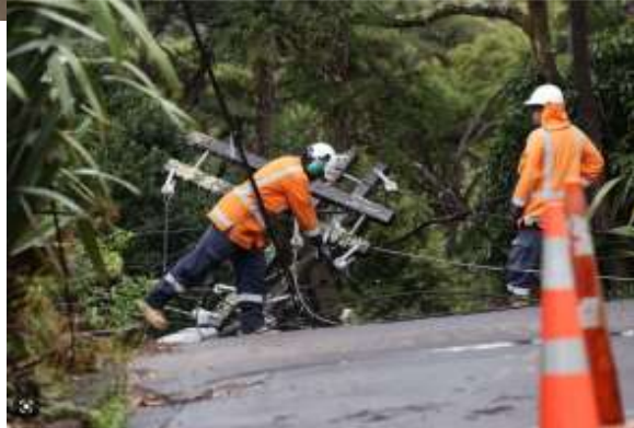
Catrina's damage eats up all year's lines repair budget | BusinessDesk
